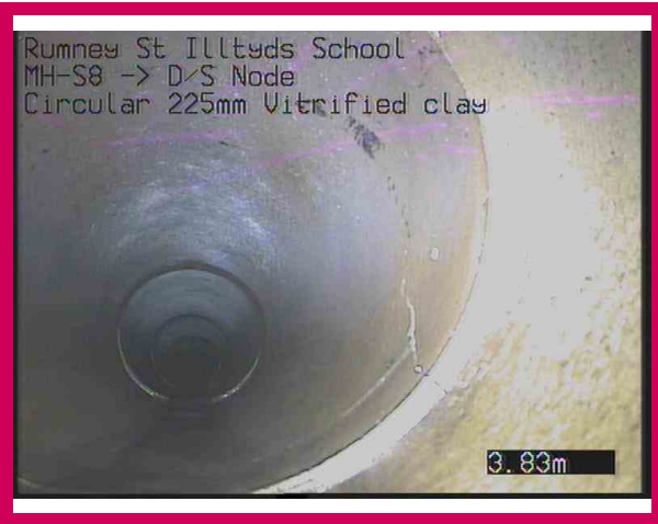
1, 00:00:46, 3.83 m Fracture, circumferential at joint from 2 o'clock to 5 o'clock
