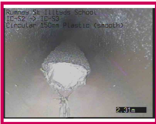
3, 00:00:50, 2.31 m Settled deposits, coarse, 30% cross-sectional area loss, start
