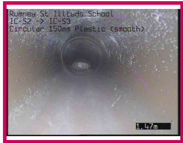
2, 00:00:32, 1.47 m Settled deposits, coarse, 5% cross-sectional area loss, finish
