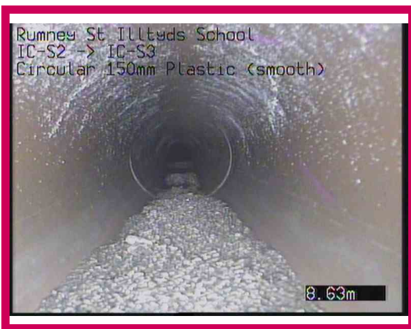
5, 00:03:55, 8.63 m Settled deposits, coarse, 30% cross-sectional area loss, finish
