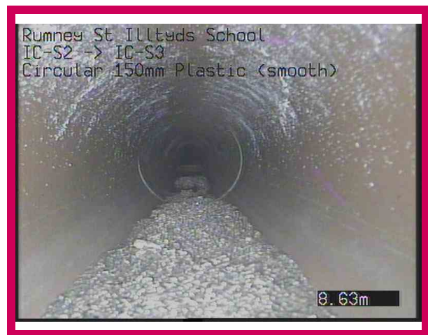
6, 00:03:55, 8.63 m Survey abandoned, Crawler unable to push debris any further
