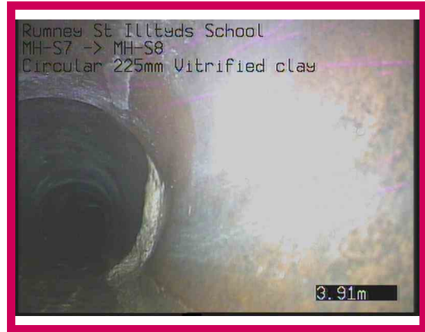
2, 00:00:42, 3.91 m Attached deposits, encrustation at joint from 2 o'clock to 10 o'clock, 5% cross-sectional area loss
