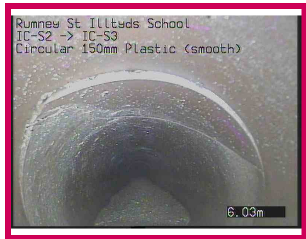
4, 00:02:04, 6.03 m Fracture, circumferential from 9 o'clock to 3 o'clock
