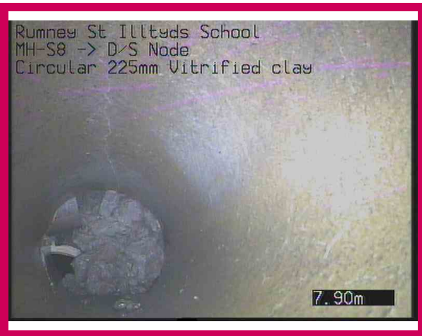
3, 00:01:23, 7.90 m Fracture, multiple from 12 o'clock to 12 o'clock
