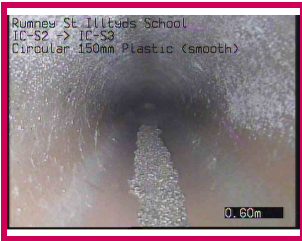
1, 00:00:21, 0.60 m Settled deposits, coarse, 5% cross-sectional area loss, start
