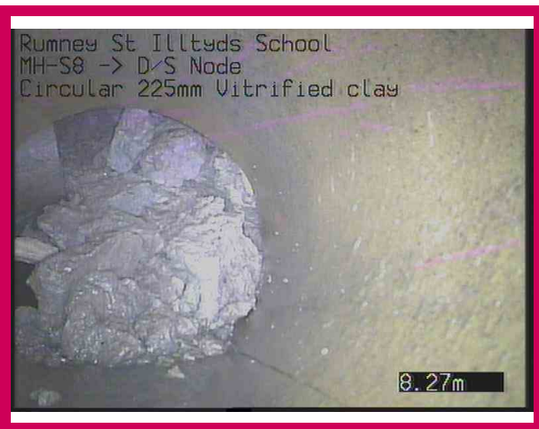
5, 00:01:37, 8.27 m Survey abandoned, Camera unable to pass collapsed pipework
