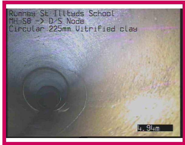
2, 00:01:00, 4.94 m Fracture spiral from 2 o'clock to 6 o'clock
