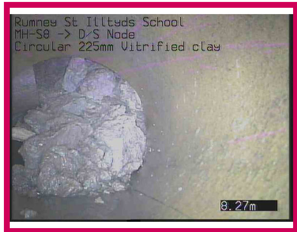
4, 00:01:35, 8.27 m Collapsed drain or sewer
